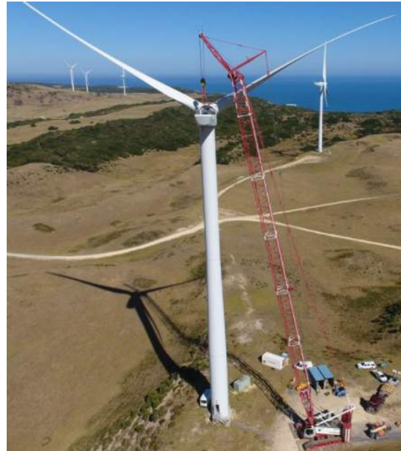
Wind turbines are decommissioned in the exact reverse of how they are constructed, with cranes removing components from the top down.
