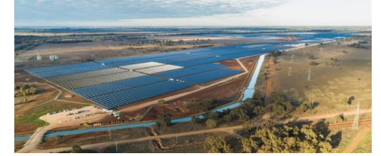
COLEAMBALLY SOLAR FARM
